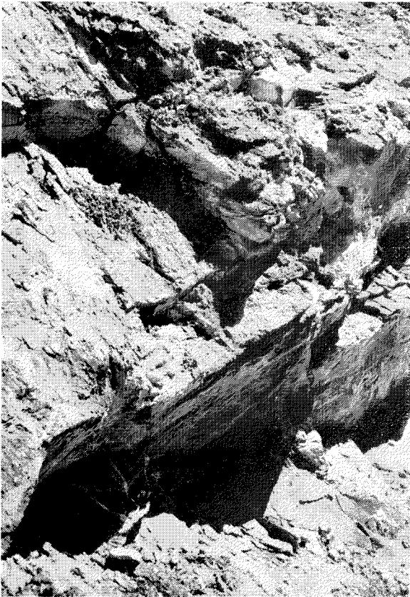
A—Overhang at 1 mile 69.5 chains. The highly to completely weathered gneiss, collapsing into the cutting on the sheet joint surface, is defined by joints striking in the same direction as the sheet joints, and dipping at right angles to it. Seepage on main sheet joint initiating movement.
