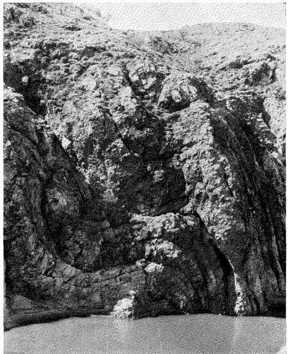
C—Folding showing well developed gapes immediately upstream of centre line, left abutment ; F 1147.
