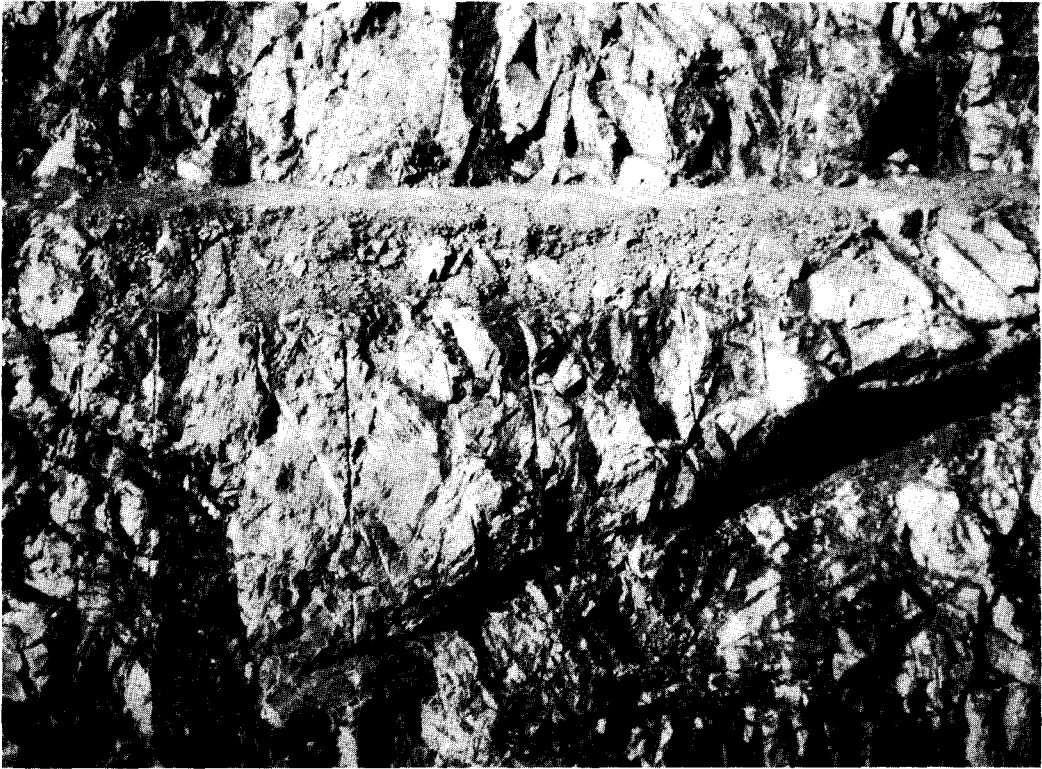
A. A steeply dipping joint plane has caused overbreak at the toe of a batter. Note also the loss of the berm edge, now filled with rubble, because of numerous blasting cycles; FN 1241.
