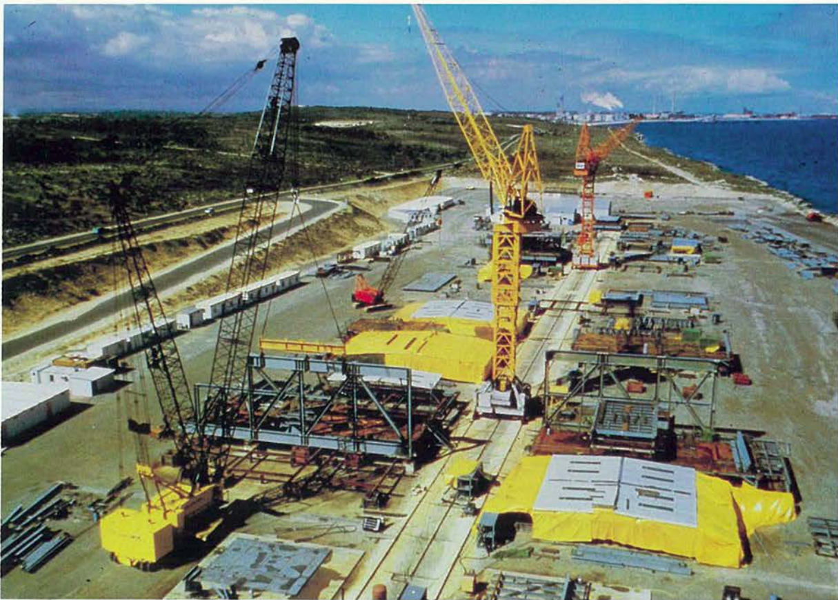
Constructing modules at Jervoise Bay for the Northwest Shelf gas production platform.
