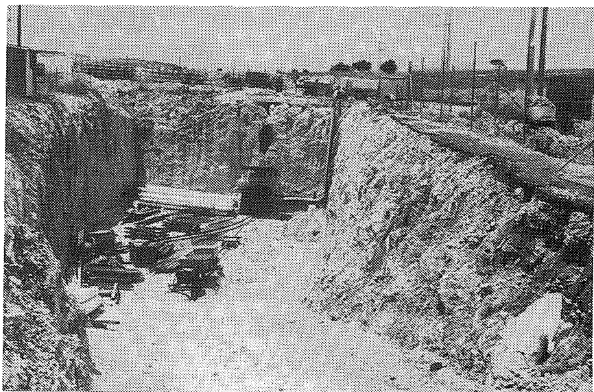
In 1983 engineering geology investigations were conducted on the Ahoy Tunnel, constructed for the Point Peron waste disposal project.
