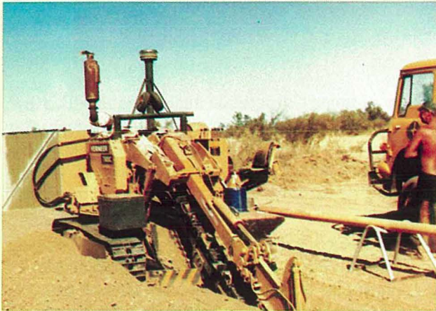
Trenching prior to burial of the 28.5 km-long pipeline linking the Blina oil production field to the Erskine storage depot on Great Northern Highway.
