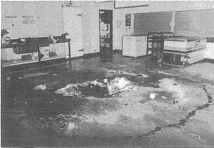
Scene of wilful damage where scientific techniques were used to assist Police investigations.
