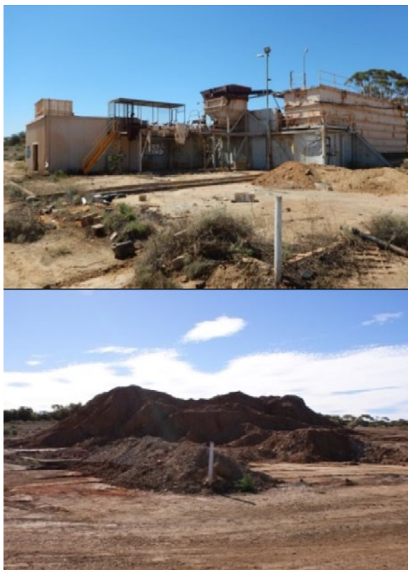
Figure 10: Pro-Force processing plant before (top) and after (below) removal.
