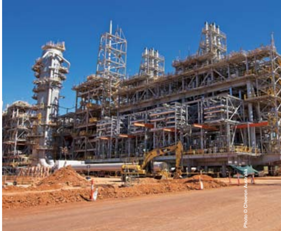
Carbon dioxide compression module, Gorgon Project
