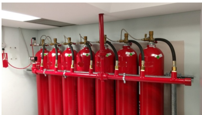
A fire-suppression system's gas storage cylinders.
