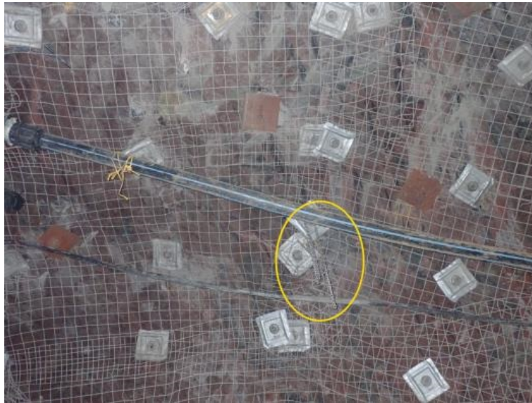
View of the failed chain installed to secure the air line to the backs.
