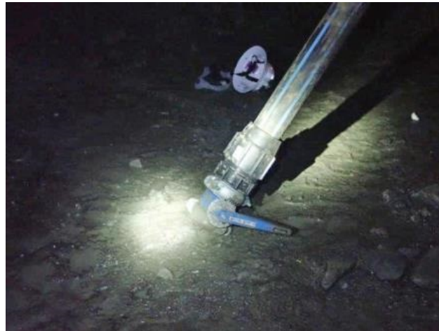
View of the failed coupling.
