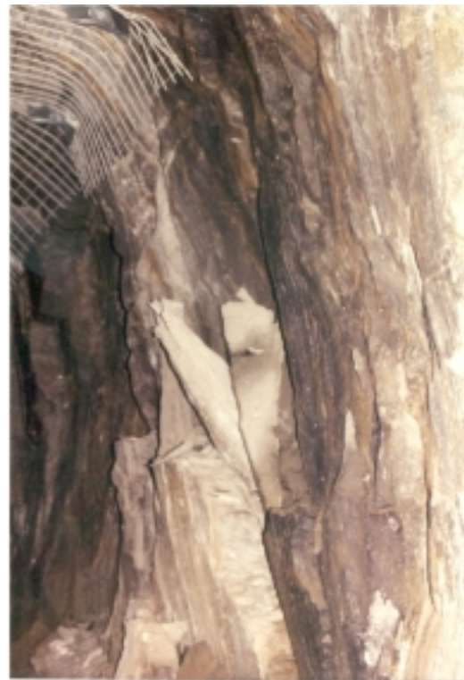
An experienced miner would know the importance of scaling loose rocks on sidewalls and be better able to assess whether scaling is necessary
