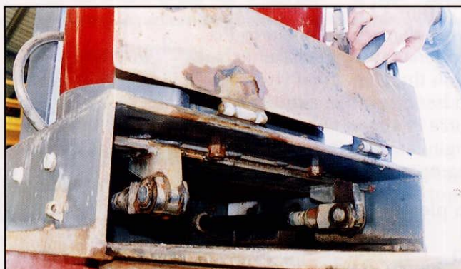
Area inside the bottom of the cyclone where the knife valve severed the victim's thumb.
