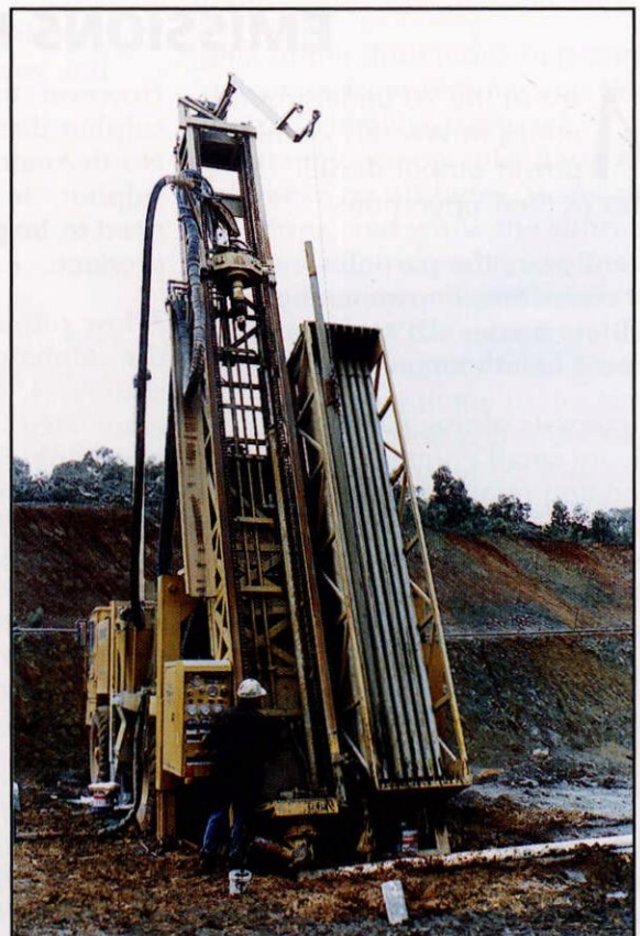
The drill rig from the lefthand side of the rig towards the rear.
