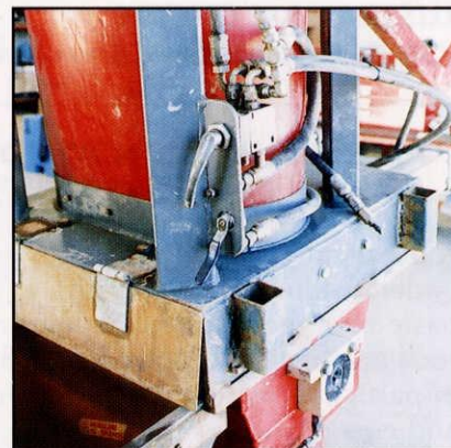
Control arrangements on cyclone.
