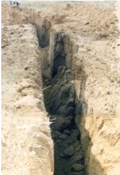
View of the costean wall collapse that fatally injured an exploration worker in 1986.
