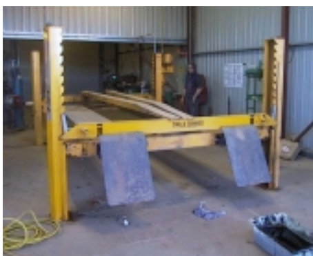
Overall view of a 4-post hoist
