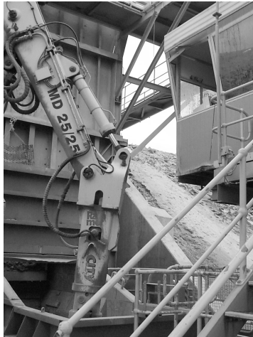
Rock breaker, jaw crusher and control cabin
