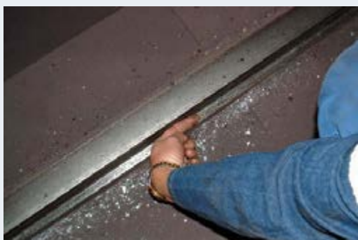
Severe rail wear (thickness of a finger). The shards of material were from the rail and the crane wheel flange.
