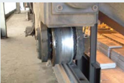
Crane wheel inner flange worn off.
