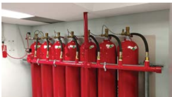
A fire-suppression system's gas storage cylinders.
