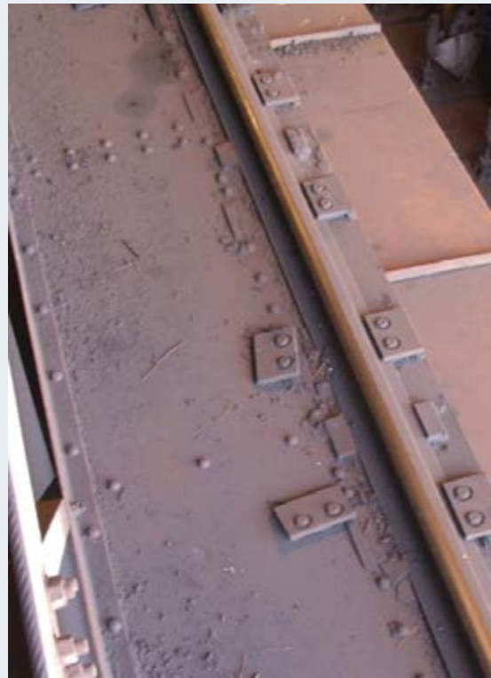
Rail clips broken off.
