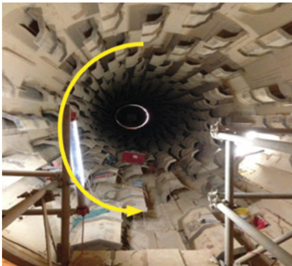
Inside view of the rotary kiln dryer showing lifter plates welded to the shell and the direction of shell rotation during incident
