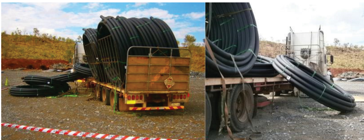
Rolls of poly pipe that fell after the pack's binding strap was cut. The driver fell to the right side of the trailer after being caught in a sliding roll. Note the intact packs of poly pipe rolls at back of trailer showing the arrangement of restraints
