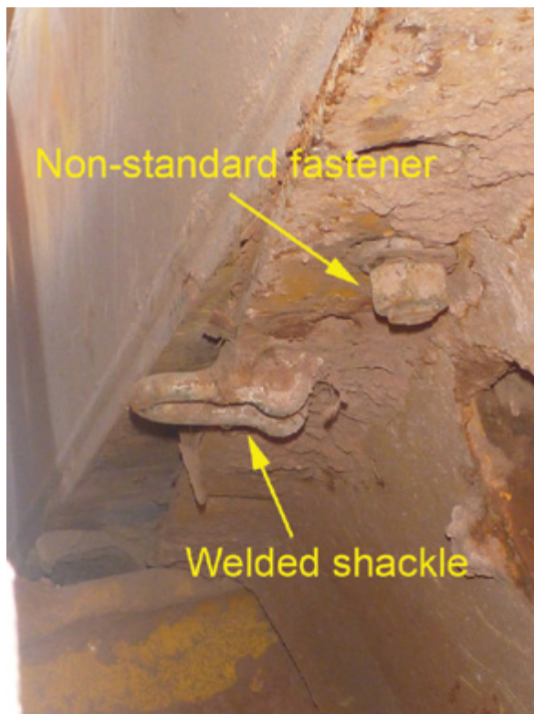
View from below showing non-OEM modifications to the right-hand side of the belly plate
