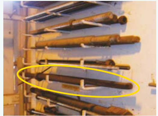
▲ Threaded bar used as a puller – what is its rated capacity?
