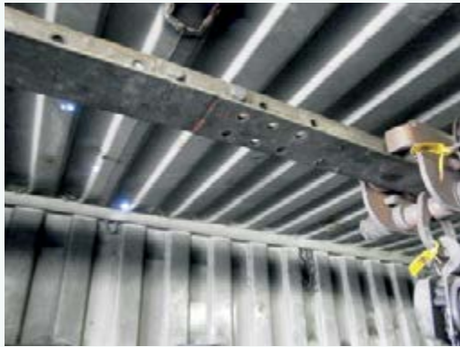
▲ Improvised overhead crane – how was the SWL determined, if at all?
