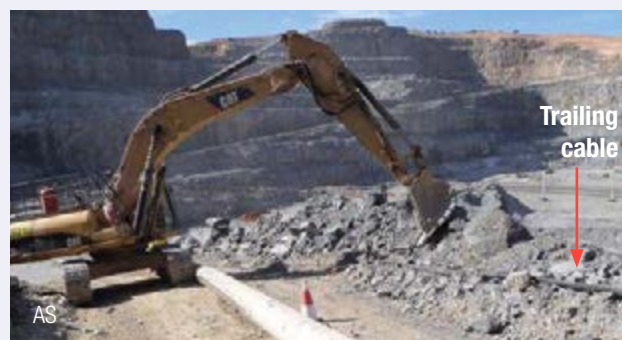
Figure 1 Trailing cable damaged by excavator
