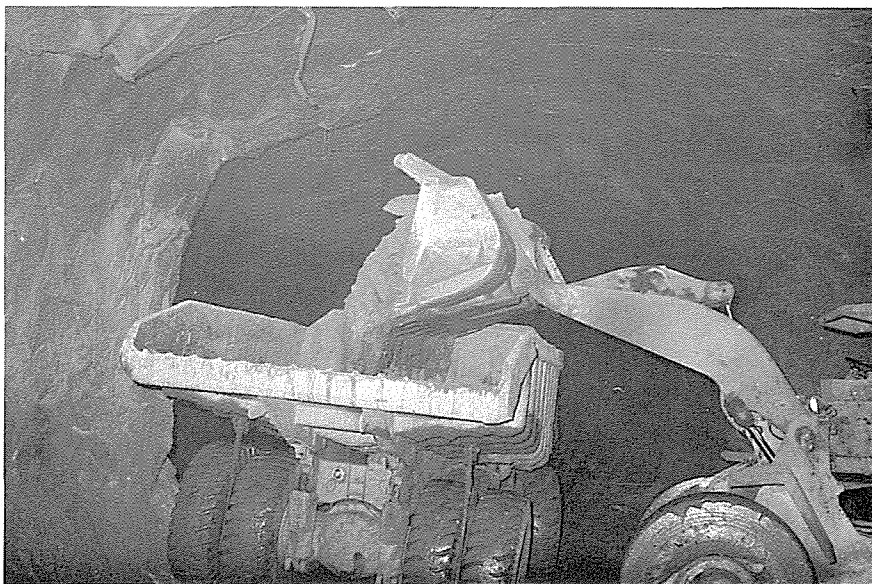
980C Caterpillar Loader and 769B Caterpillar Truck. 18 level No.11 Mill Hole, Mt Charlotte
