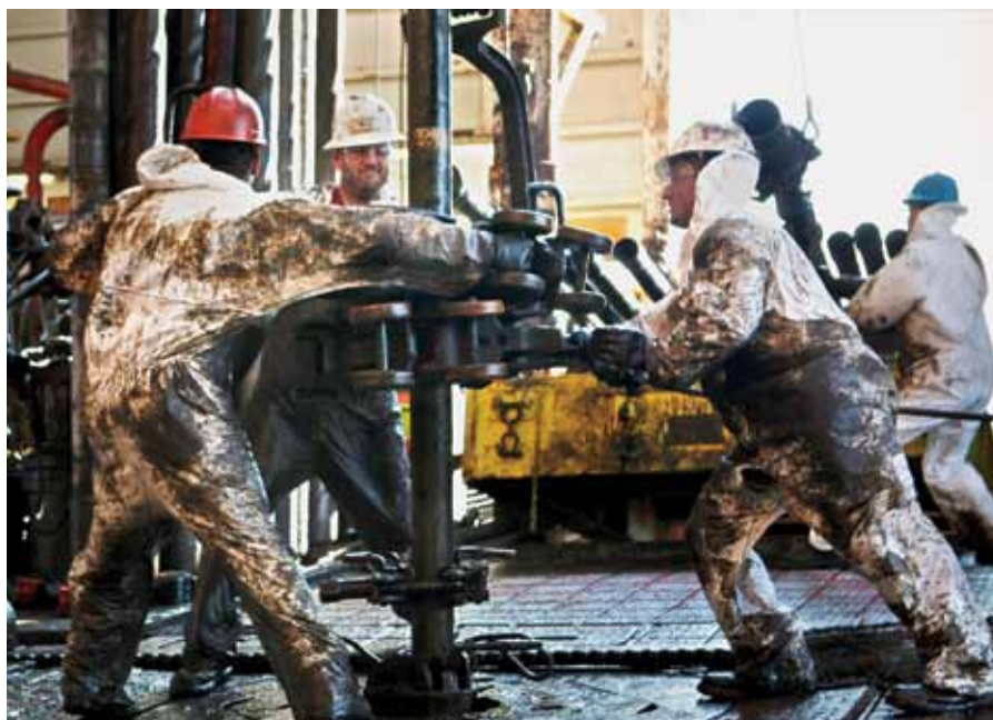
Drillers at work on the Jack Bates (Photo courtesy of Kai Photography and Hess Exploration)
