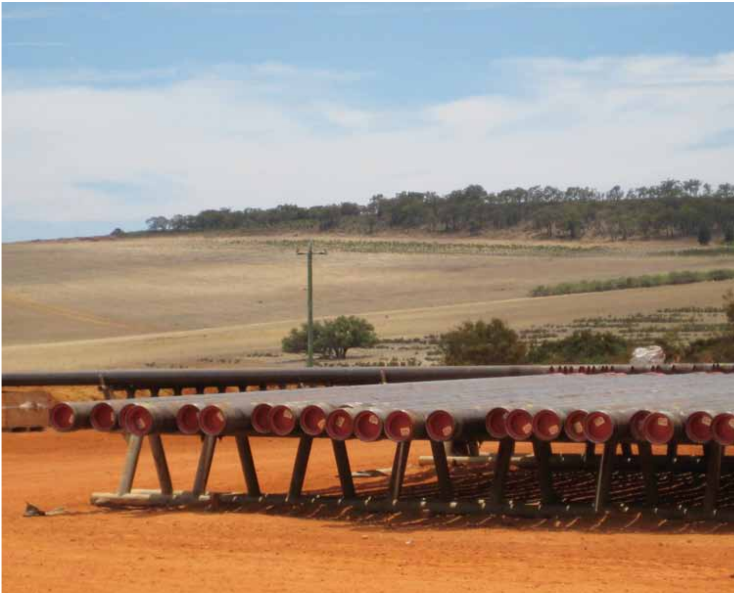
Drill pipe ready to go in the onshore Perth Basin (Photo courtesy of Karina Jonasson)
