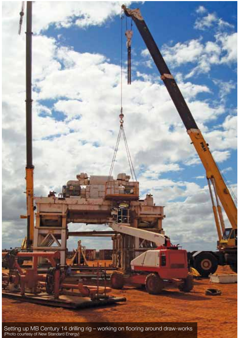
Setting up MB Century 14 drilling rig – mast pinning (Photo courtesy of New Standard Energy)
