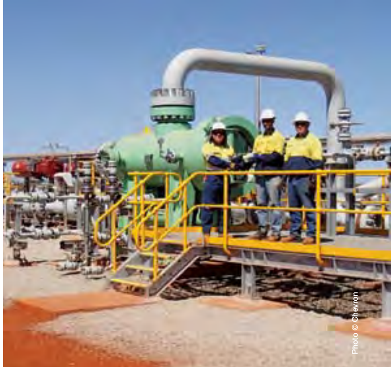
The domestic gas meter station for the Gorgon Project will supply gas to the DBNGP
