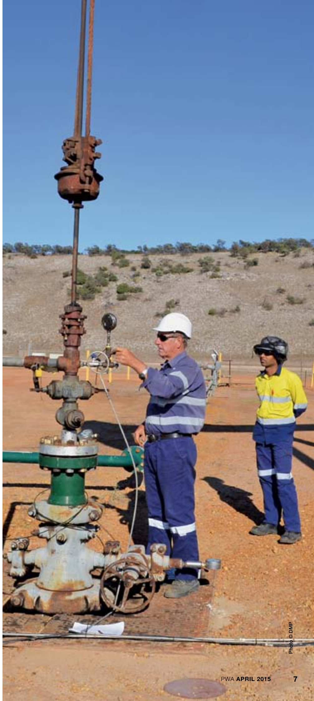
Petroleum Division inspector on a well integrity inspection at the Dongara field
