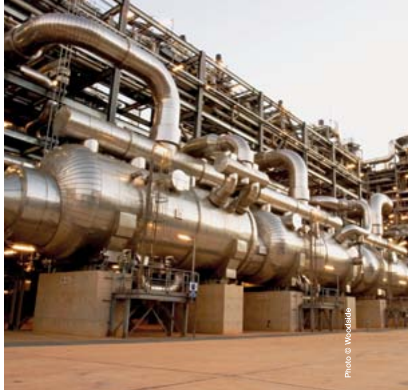
NWS domestic gas plant at Karratha
