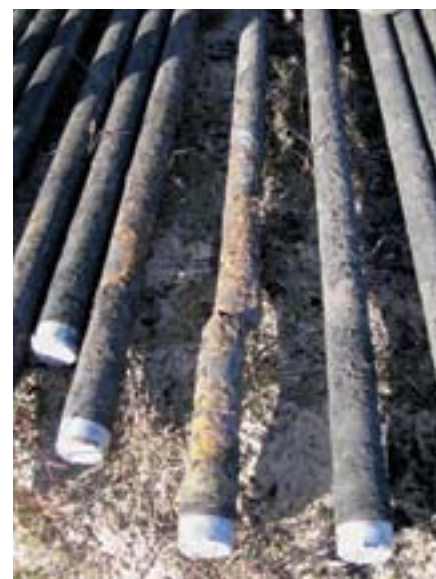
Figure 3. Tubing that has twisted due to corrosion (Source: DMP)
