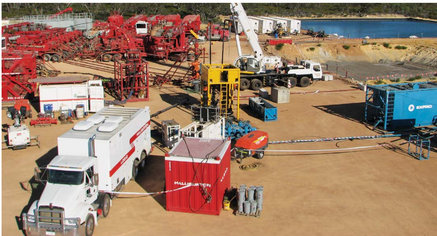
Arrowsmith 2 well in the northern Perth Basin undergoing hydraulic fracture stimulation. Source: Norwest Energy NL
