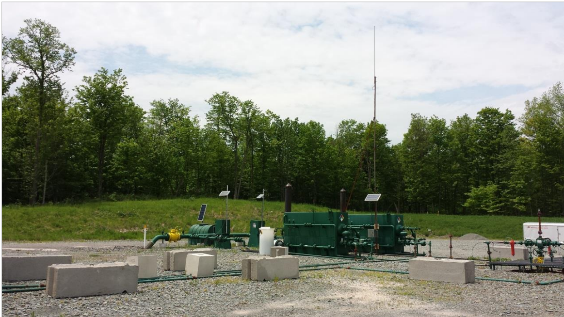
Figure 15. Remediated onshore shale gas well on private land in Dimock, Pennsylvania (from different angles)
