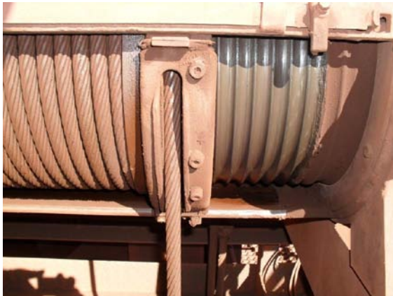
Figure 1 Undamaged metal rope guide on the hoist winch of a Demag crane model P416H22L
