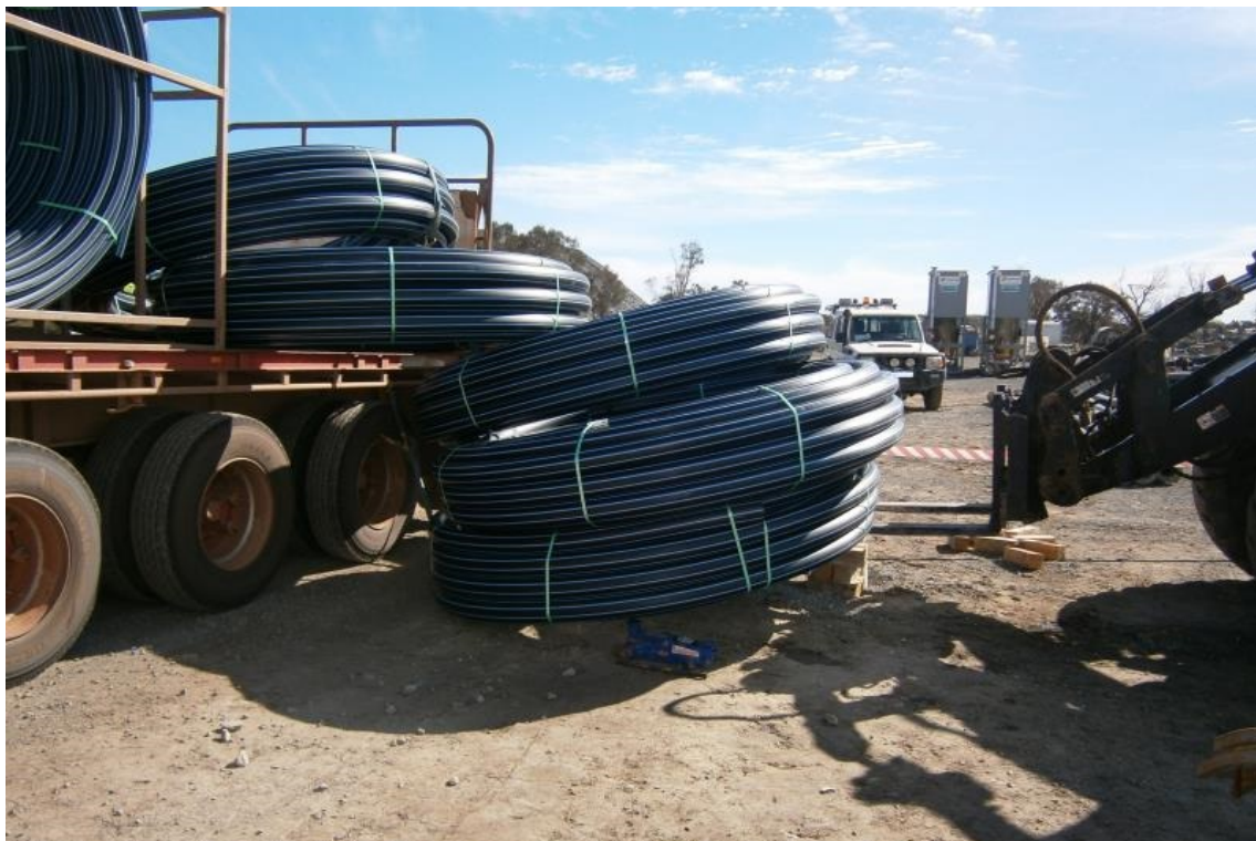
Position of poly pipe after the incident. The forklift and hydraulic jacks were used to move the poly pipe to access the underground operator trapped beneath.
