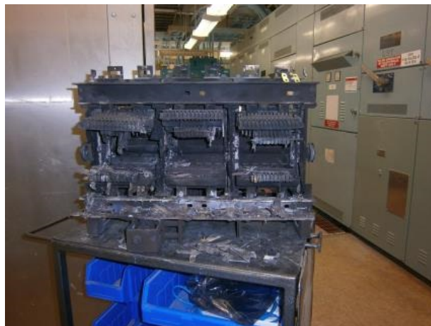
Damage to 4,000 A switch following incident
