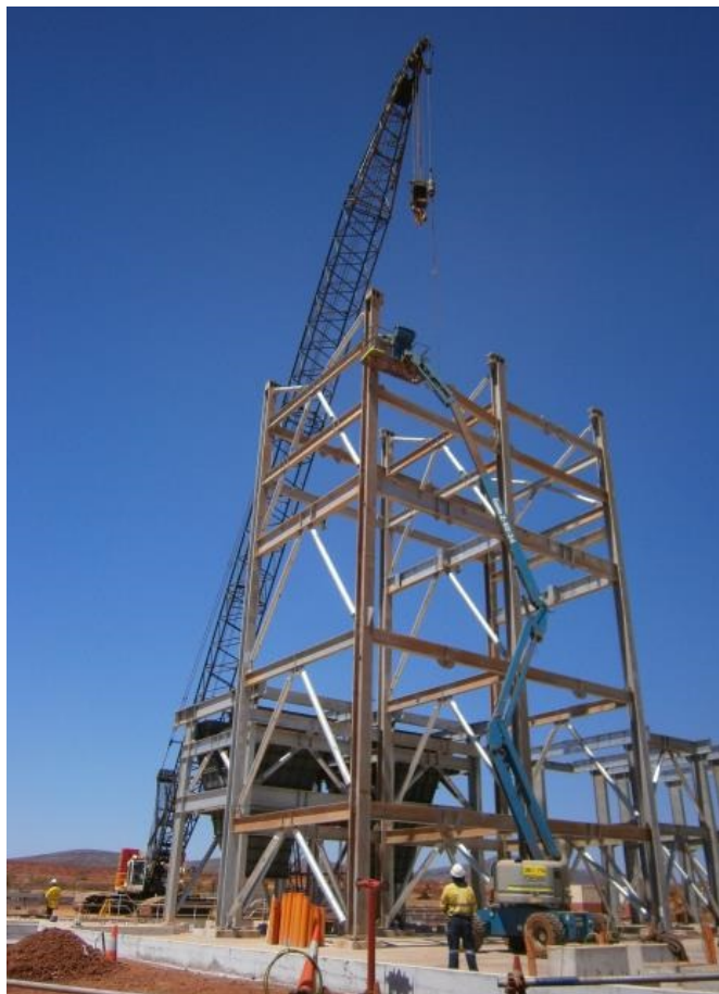
Spotter has obscured view of work being undertaken by MEWP operator and might not recognise potential for interaction with other activities
