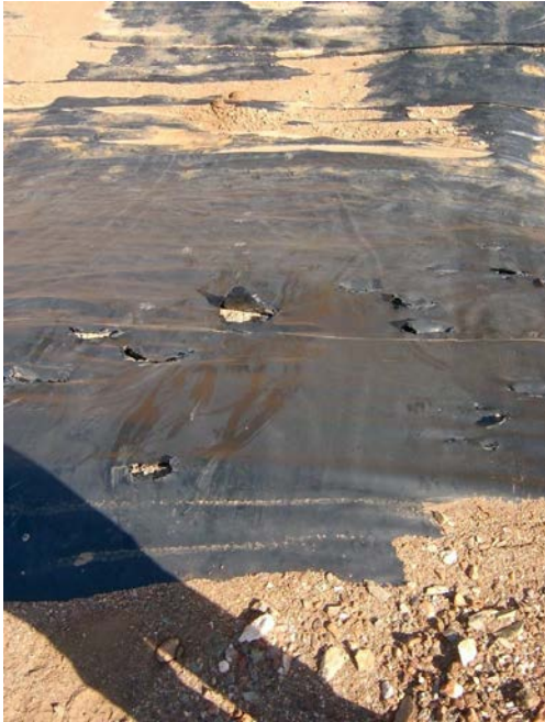
Plate 2: damaged liner from fauna attempting to climb the pond wall.
