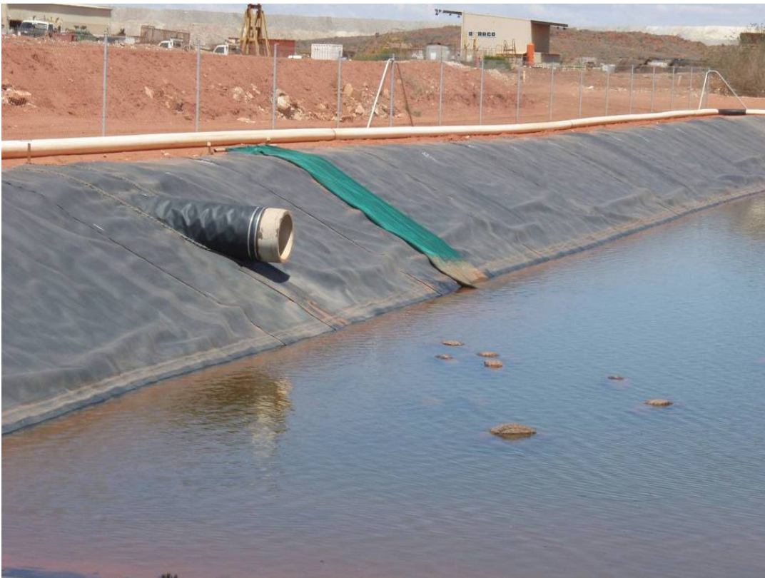
Plate 7: Shade cloth fixed to conveyor belt matting (Telfer, Newcrest Mining Ltd).
