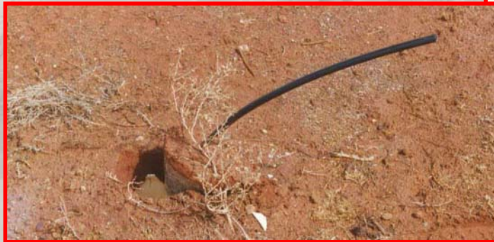
Inappropriately plugged drillhole
