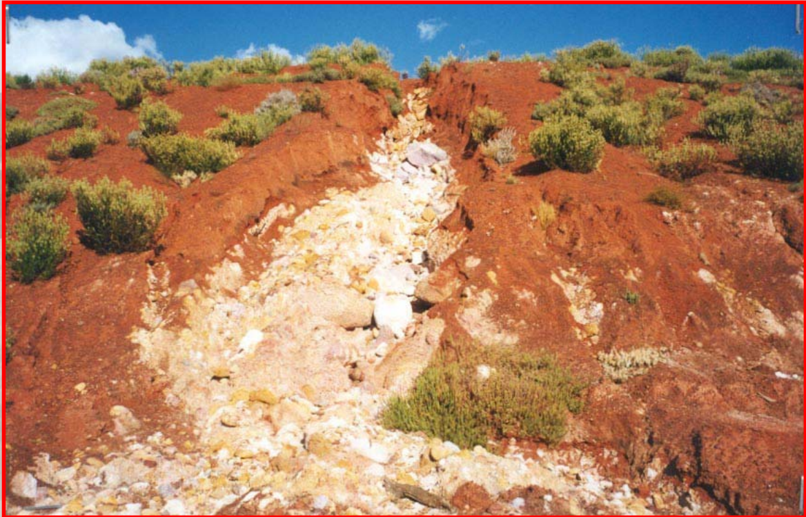
Erosion due to poorly designed water-control structures
