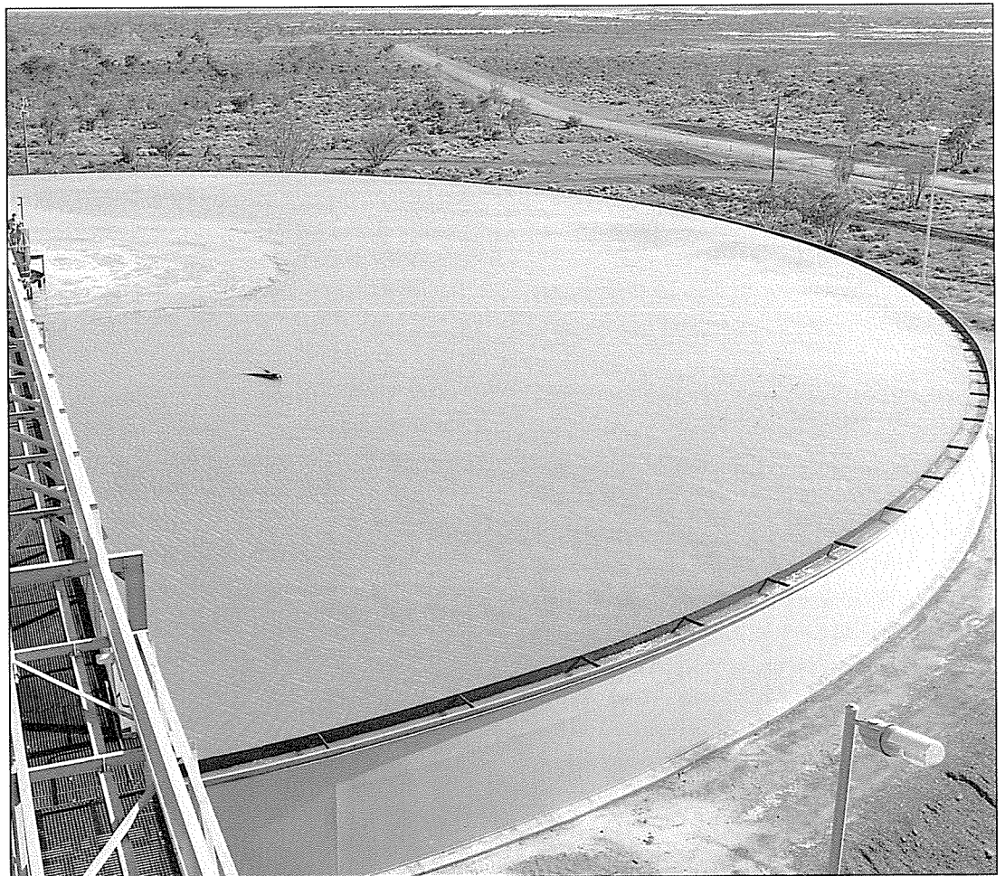
A thickening tank, part of the big Kaltails slime dump retreatment project on the southern outskirts of Kalgoorlie-Boulder.
