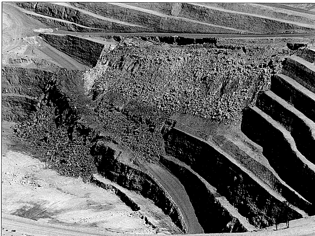
Pitwall failures, like this one in the Eastern Goldfields, proved a real headache for mining companies and the Department of Mines during 1989-90.
