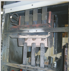
Mines Safety Significant Incident Report No. 191
