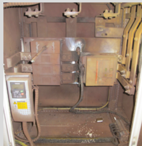
Mines Safety Significant Incident Report No. 192
