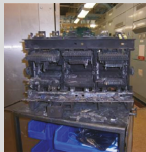
Mines Safety Significant Incident Report No. 239
