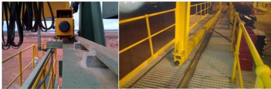
Upper carriage (left) and lower carriage (right) of semi-gantry crane following a derailment.
