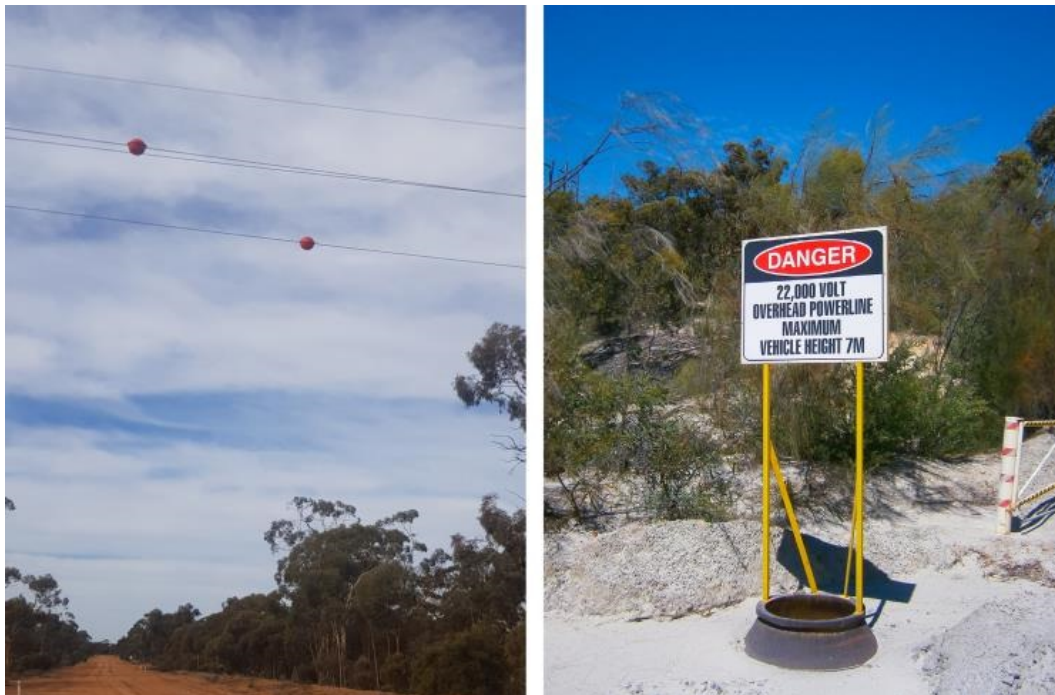
Examples of clearance indicators and signage for high voltage overhead powerlines
