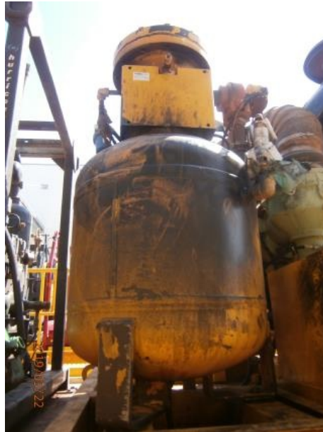
Air/oil separator vessel The carbon deposits on outside of shell indicated the venting from the safety relief valve during internal flash-over.
