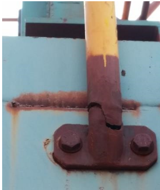
Handrail post failure after inappropriate repair. The corrosion was removed and the area painted without strengthening.
