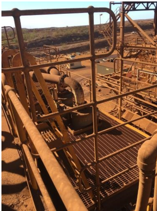
Handrails with six rails not in accordance with manufacturer's specifications of two rails.
