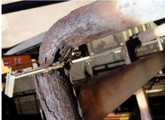
Delayed maintenance led to handrail failure.
