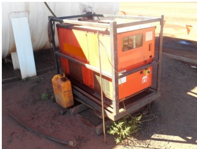
Poor housekeeping standard at a temporary generator installation.
