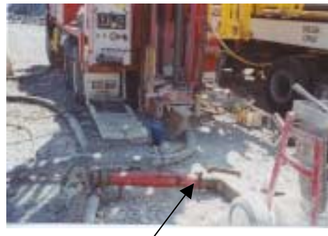
“Tile box” assembly after falling from mast.
