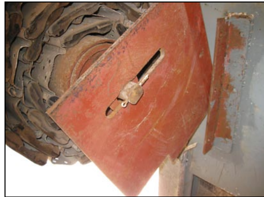
Close-up view of support bracket after incident
