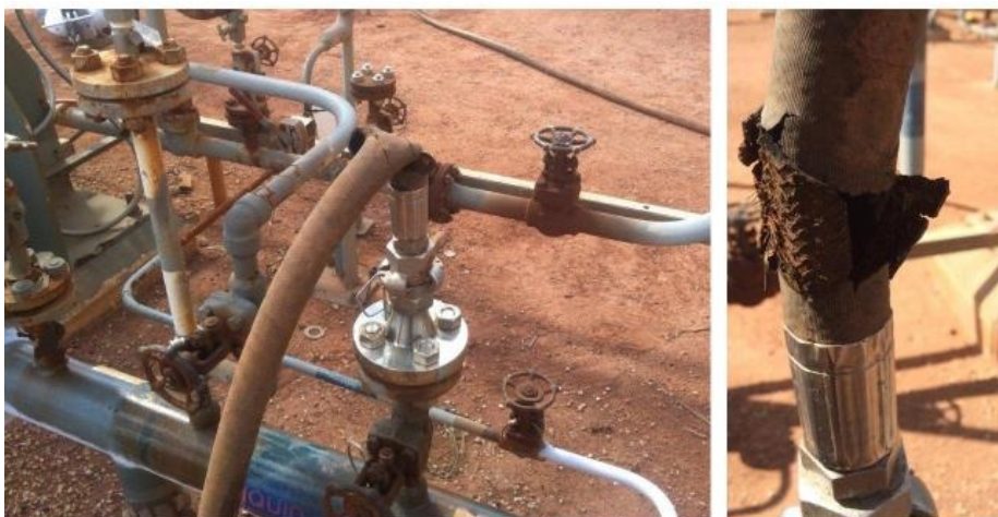
Flexible rubber hose and assembly connected to anhydrous ammonia purge point. Close up (right) shows rupture in hose above connection point
