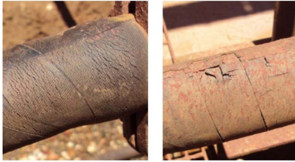
Flexible rubber hoses showing external damage. Only testing by a competent person will reveal whether the internal integrity of the hose has been compromised
