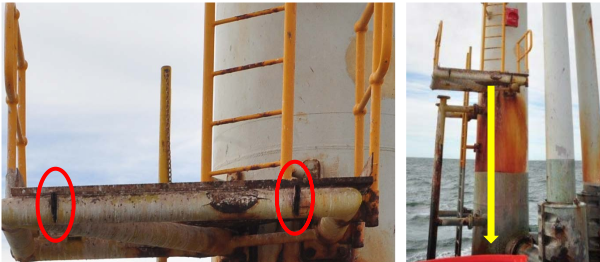
Photographs showing location of handrail attachments that failed (left) and fall path from landing (right)
