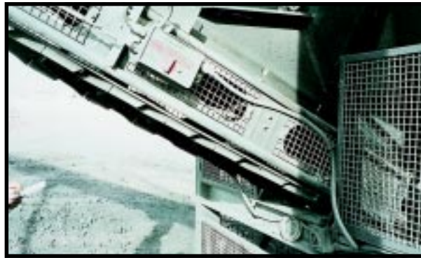
Fig (1) A very good approach to guarding except for probably the most critical nip point of all which could drag persons in to such an extent that they may not be able to reach the emergency-stop lanyard.
