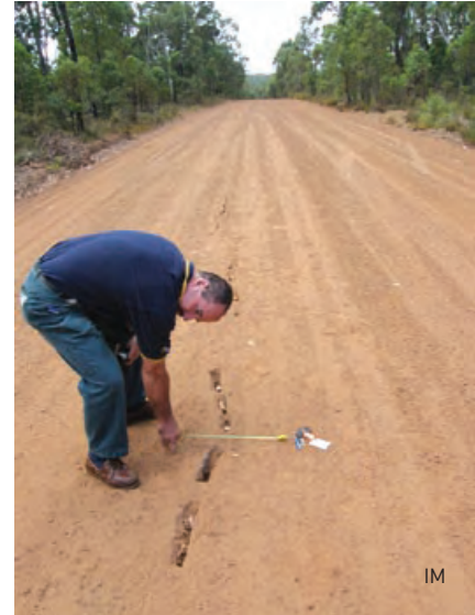
Measuring cracks on Shotts Road
