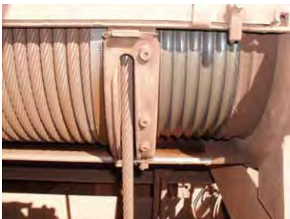
Figure 1 Undamaged metal rope guide on the hoist winch of a Demag crane model P416H22L
