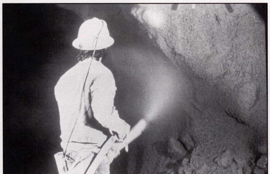
The skill and knowledge of the nozzleman is critical to the successful application of shotcrete.
