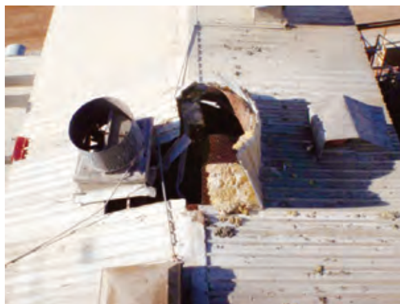
Figure 1 Damage caused when the 500 kg IPSE lid punched through the gold room roof
