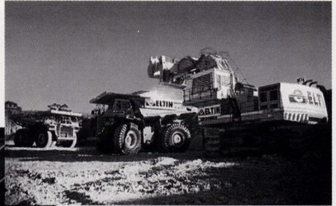
Leibherr 994 Face Shovel loading a Cat 785 dump truck. A second is waiting to load (Eltin)
