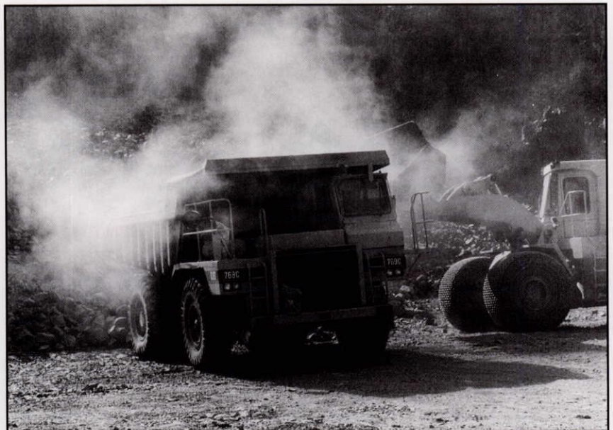
Systems must be in place to ensure levels of dust are maintained below acceptable standards.
