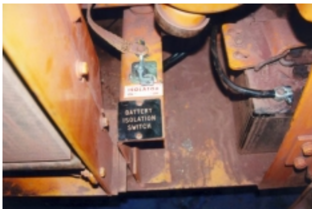
Typical mobile plant battery isolator
