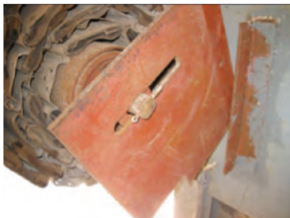
Close-up view of support bracket after incident
