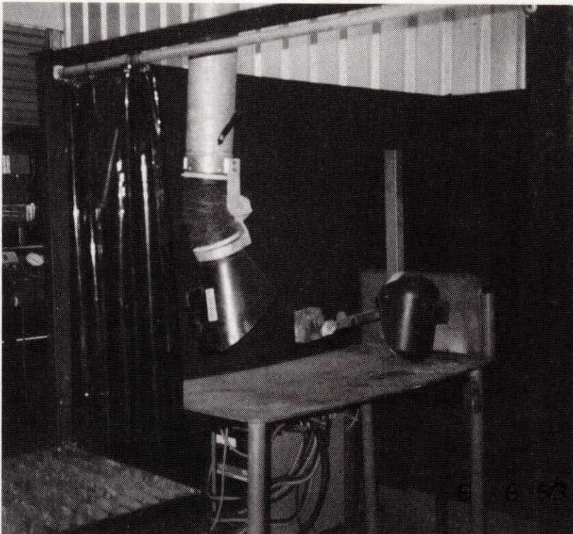
Local exhaust ventilation system at a welding station. Flexible ducting allows limited movement
